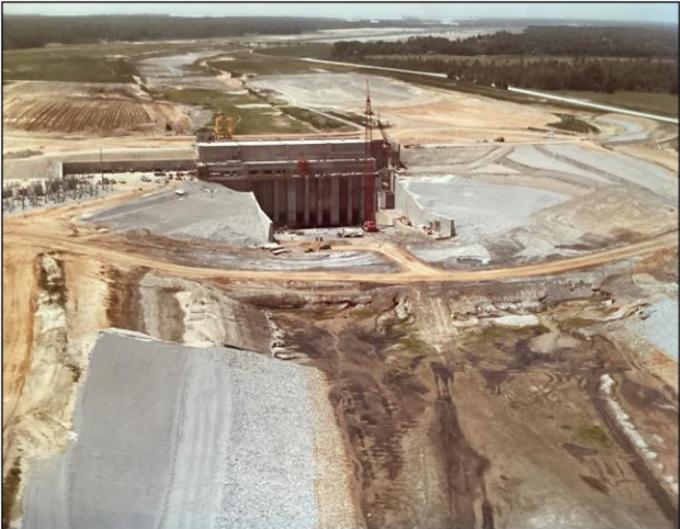
The Intake Canal to the St. Stephen Hydro Plant and into the Tailrace Canal. Project completed 1983.
